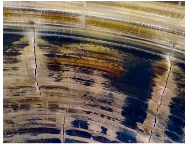
Figure 4. The scorched inner bushing surface shows long structural cracks, with the longest being 4 ft in length.
