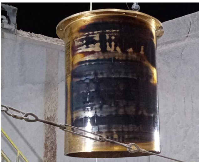
Figure 3. The outer bushing surface shows severe damage from extreme pressures, high temperatures, and burnt oil.
